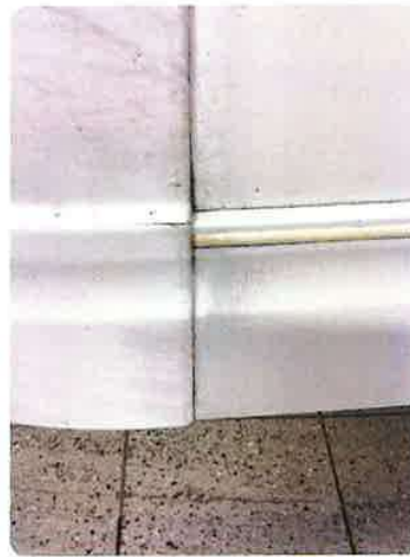
2.3 Sprekk Sprekk b-stolpedeksel v/s
